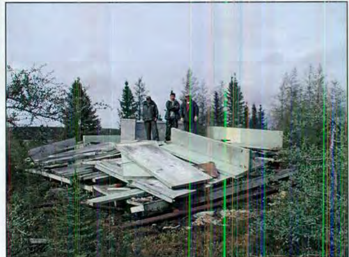
Photo 11. Site 321A (30 May 2001). State of building. Attempt to stabilize the building. Debris from the demolition.
