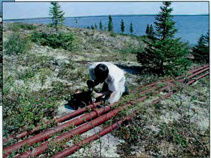
Photo 18. Section of pipe and flexible hoses reaching to the lake and dismantling the pipeline at site 318A (28 May 2001).
