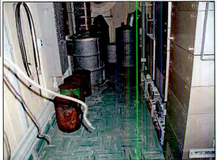
Photo 14. Transporting containers of putty at site 315 to be stored in the main building (13 October 2001).
