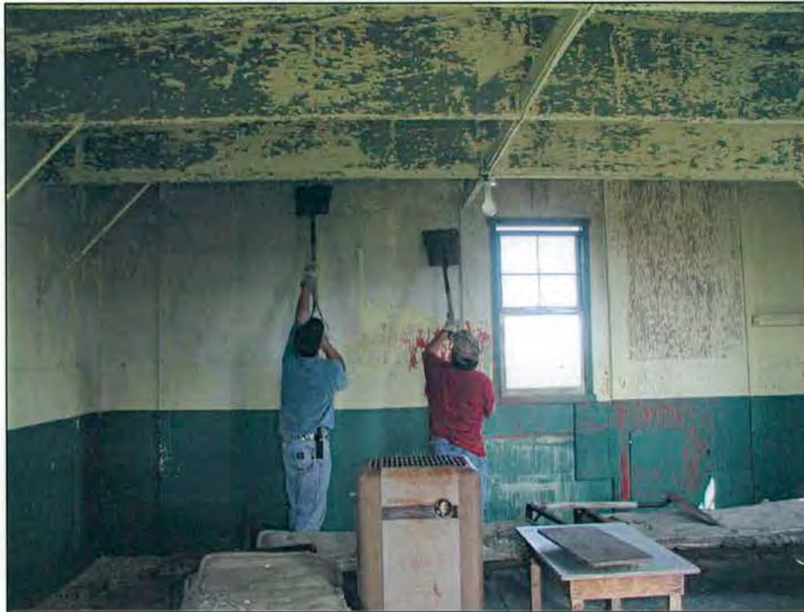
Photo 12. Scraping paint from the walls inside the survival shelter at site 315 (25 May 2001).
