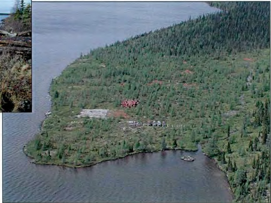
Photo 10. Aerial view of site 303A before (top, right; 11 June 2001) and following (bottom, right; 17 June 2001) completion of clean-up work. (Top and bottom, left) View of the dock before and after it was removed from the lake (17 October 2001).
